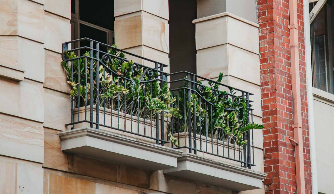
An example of a West facing residential balcony planter using Zig Zag plants
