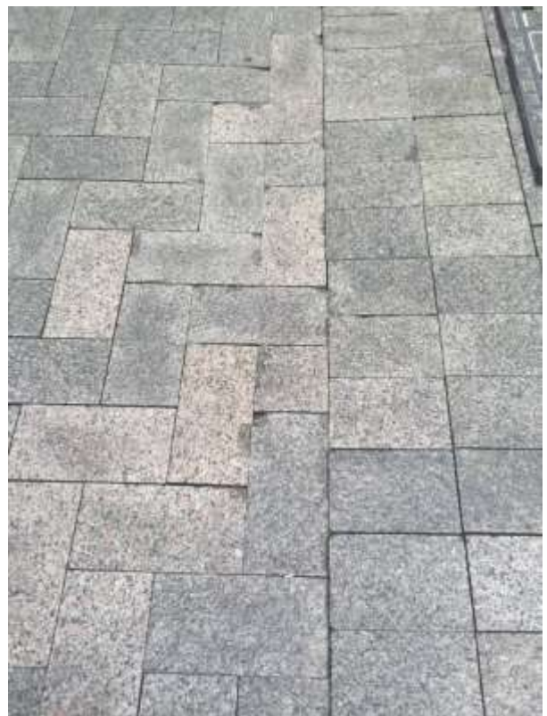
Chipped paver – Trip Hazard
