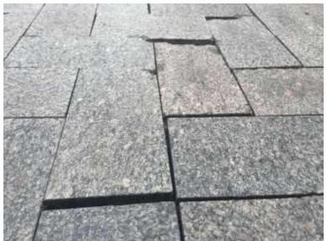
Trip hazard - Dislodged
