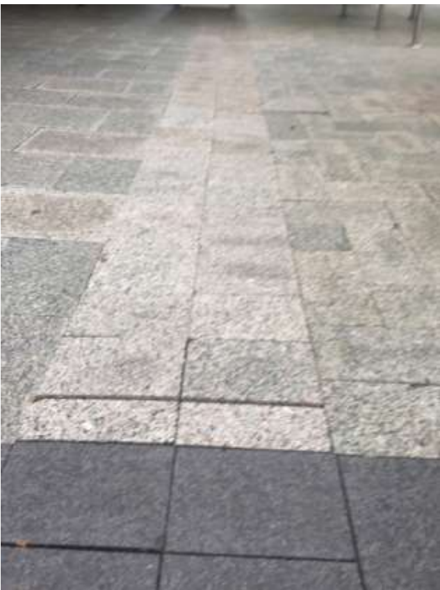
Missalignment - Trip hazard
