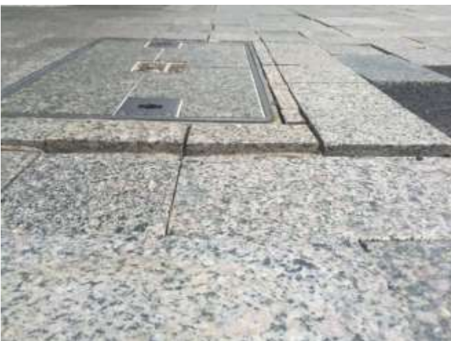
Trip hazard – Dislodged
