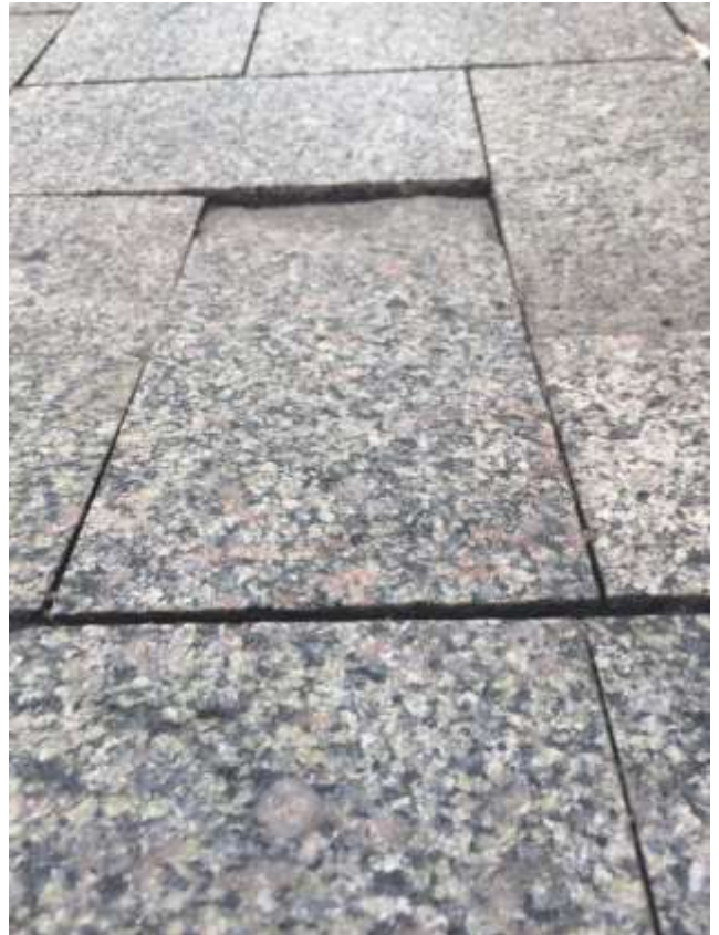
Chipped – Trip hazard
