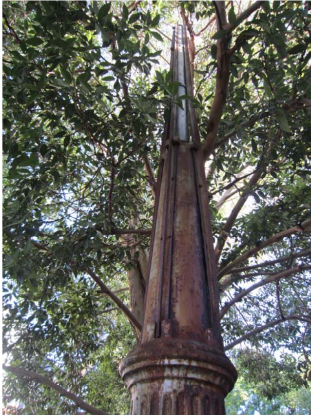
P23762 Sewerage Vent, East Perth ; Steel support brace to ventilation pipe ; Karina Williams 06 Feb 2014
