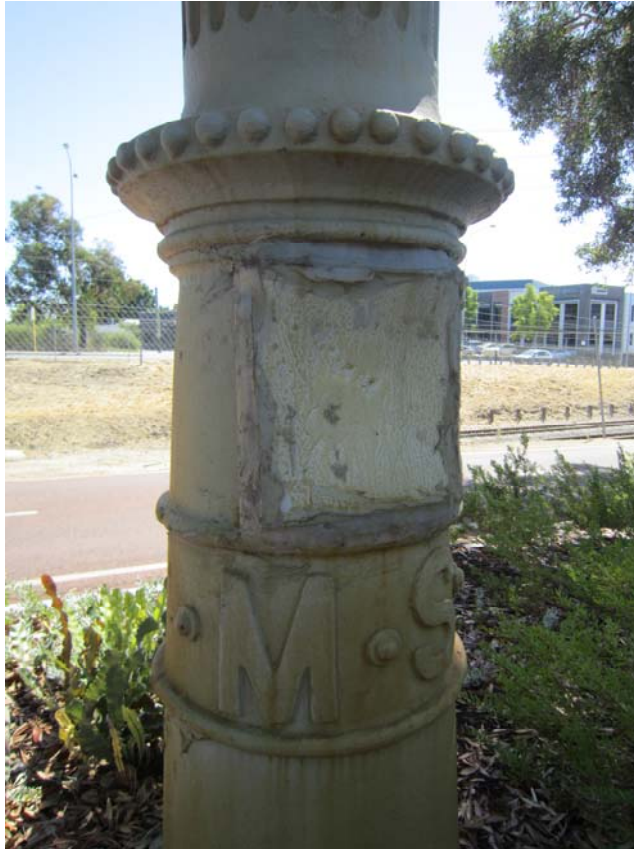
P23738 Sewerage Vent, West Perth ; Detail; M.S lettering and access panel ; Karina Williams 07 Feb 2014
