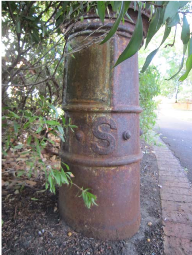
P23762 Sewerage Vent, East Perth ; Detail; cast iron base, lettering and access panel ; Karina Williams 06 Feb 2014
