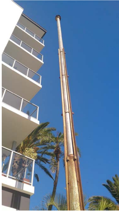
P23782 Sewerage Vent, Princess Margaret Hospital, West Perth ; View along vent pipe ; Sian Ferraz 21 Aug 2013
