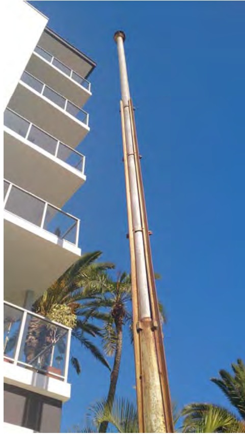
P23782 Sewerage Vent, Princess Margaret Hospital, West Perth ; View along vent pipe ; Sian Ferraz 21 Aug 2013
