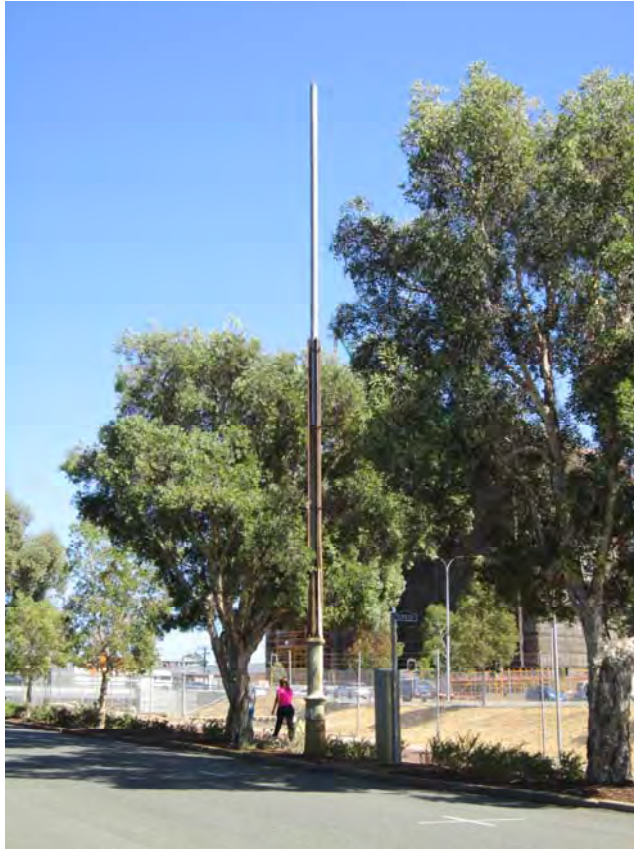
P23738 Sewerage Vent, West Perth ; View across Arthur Street, looking north ; Karina Williams 07 Feb 2014
