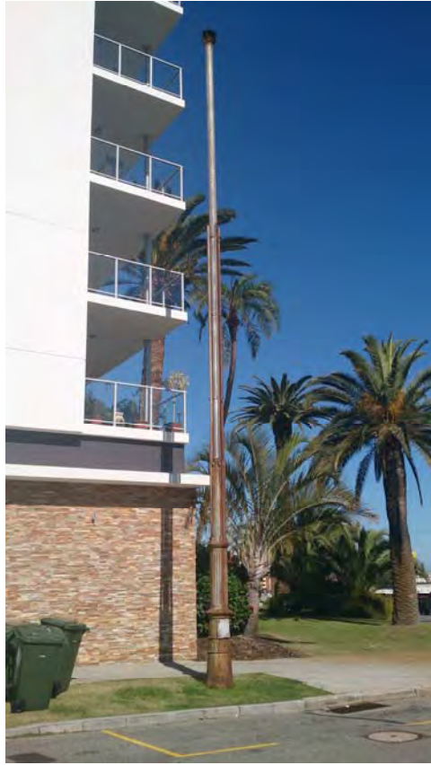
P23782 Sewerage Vent, Princess Margaret Hospital, West Perth ; View across Cook Street, looking south ; Sian Ferraz 21 Aug 2013
