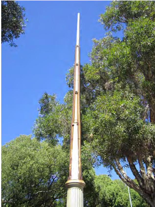
P23738 Sewerage Vent, West Perth ; Detail; support structure and top of vent ; Karina Williams 07 Feb 2014
