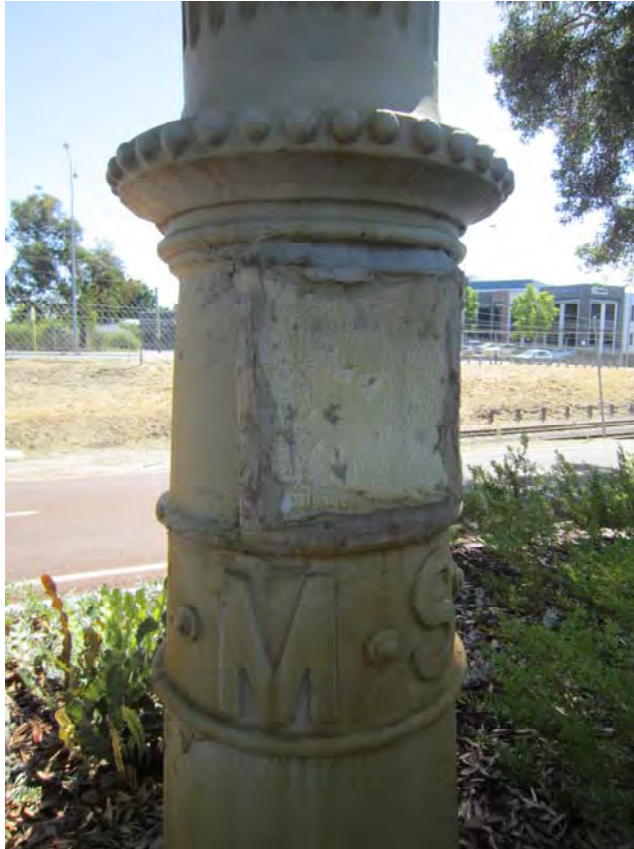
P23738 Sewerage Vent, West Perth ; Detail; M.S lettering and access panel ; Karina Williams 07 Feb 2014
