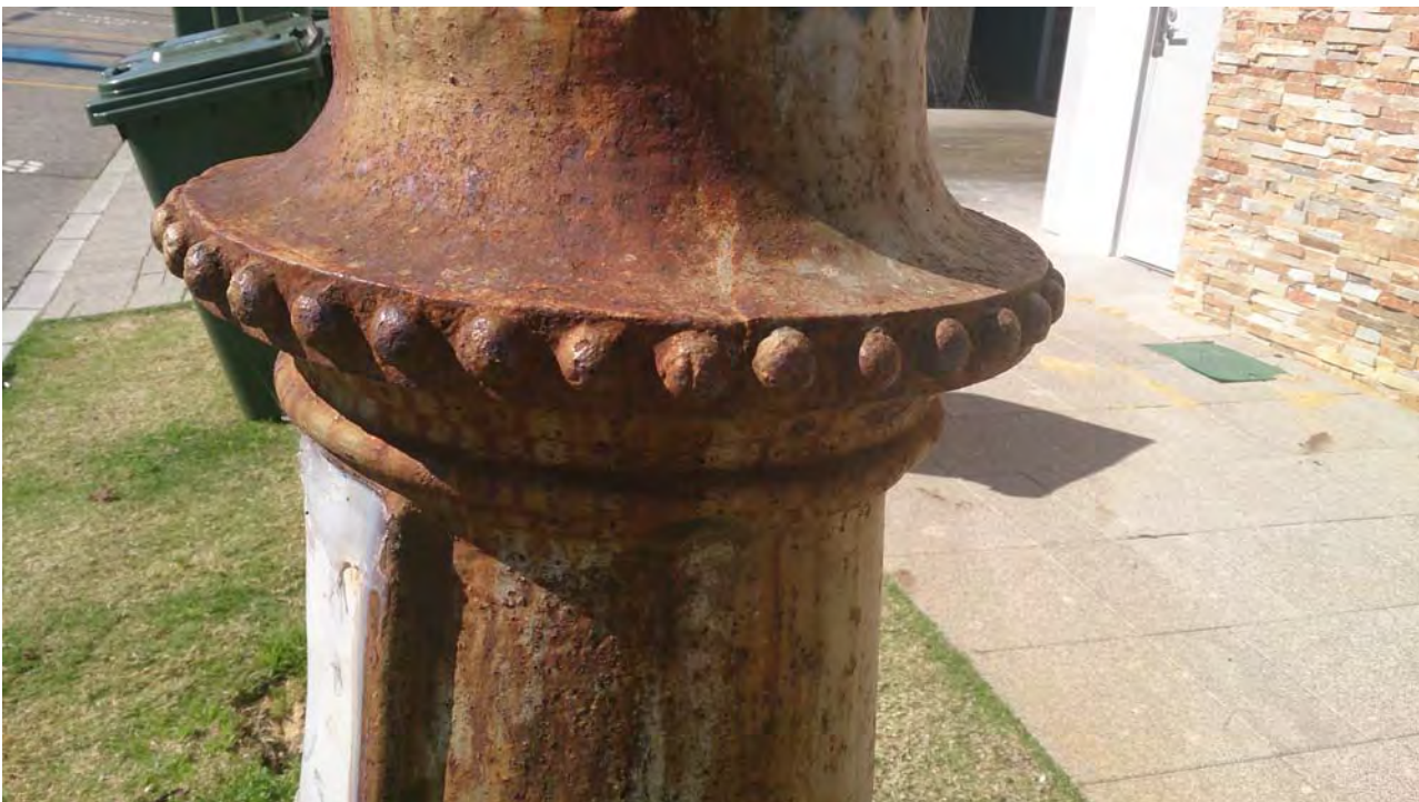
P23782 Sewerage Vent, Princess Margaret Hospital, West Perth ; Detail of Cast Iron base ; Sian Ferraz 21 Aug 2013
