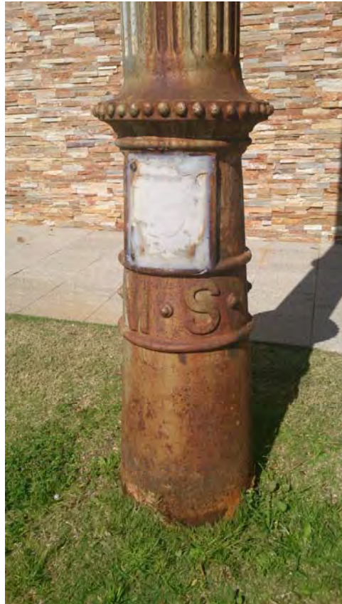
P23782 Sewerage Vent, Princess Margaret Hospital, West Perth ; View of Cast Iron base showing 'M.S' lettering ; Sian Ferraz 21 Aug 2013
