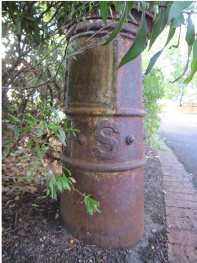
P23762 Sewerage Vent, East Perth ; Detail; cast iron base, lettering and access panel ; Karina Williams 06 Feb 2014
